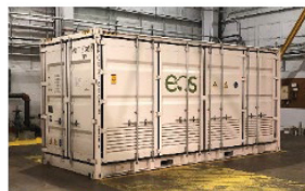
Containerized (10MW = 0.5 acres)
