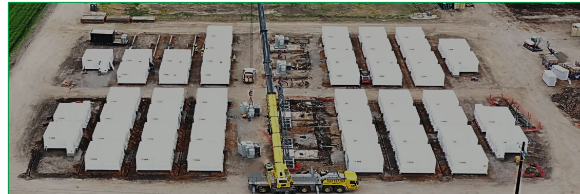
Texas - 50 MWh Stand-Alone BESS
