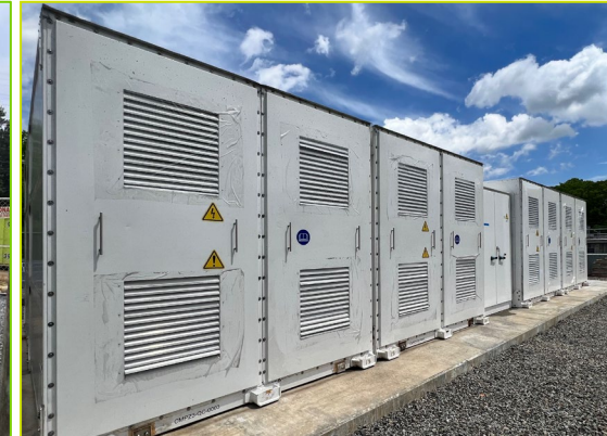
New Jersey - 2 MWh Microgrid
