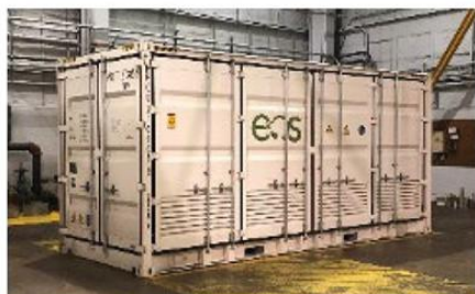
Containerized (10MW = 0.5 acres)
