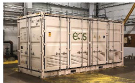
Containerized (10MW = 0.5 acres)
