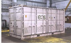
Containerized (10MW = 0.5 acres)
