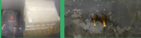
Rise in temp but no fire
