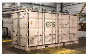
Containerized (10MW = 0.5 acres)
