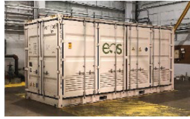
Containerized (10MW = 0.5 acres)
