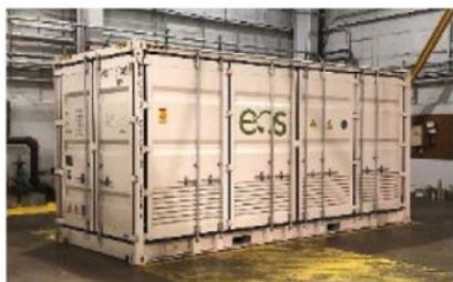
Containerized (10MW=0.5 acres)
